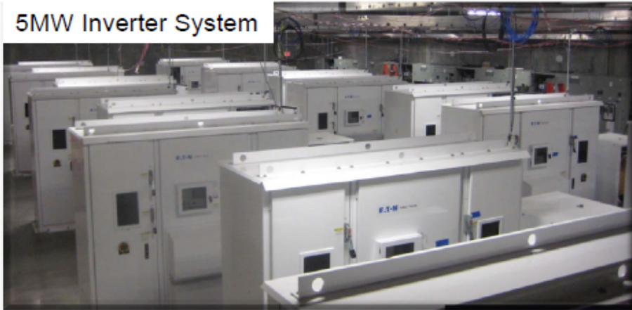
5MW Li-ion Batteries
